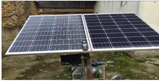
Figure 2. PV Array Testing
